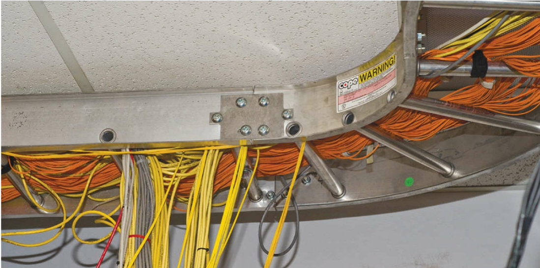
Figure 5-30 Messy cabling nightmare
