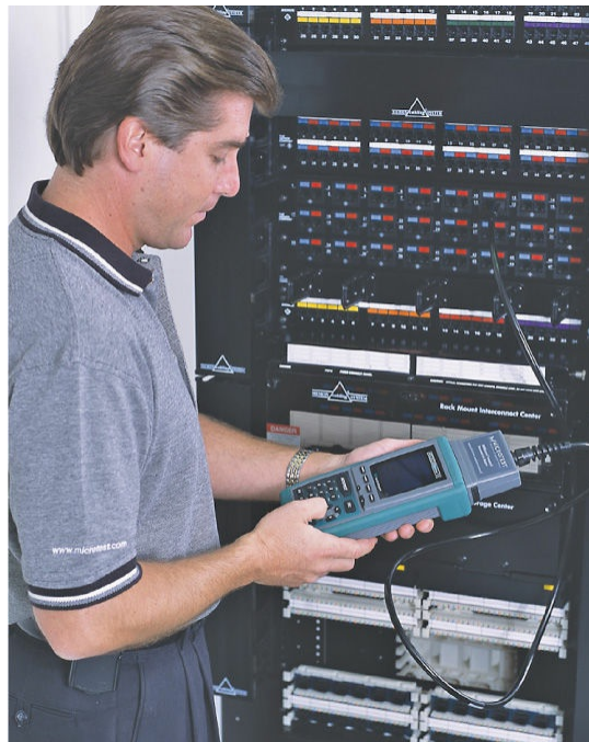
Figure 5-51 A typical cable certifier—a Microtest OMNIScanner (photo courtesy of Fluke Networks)
