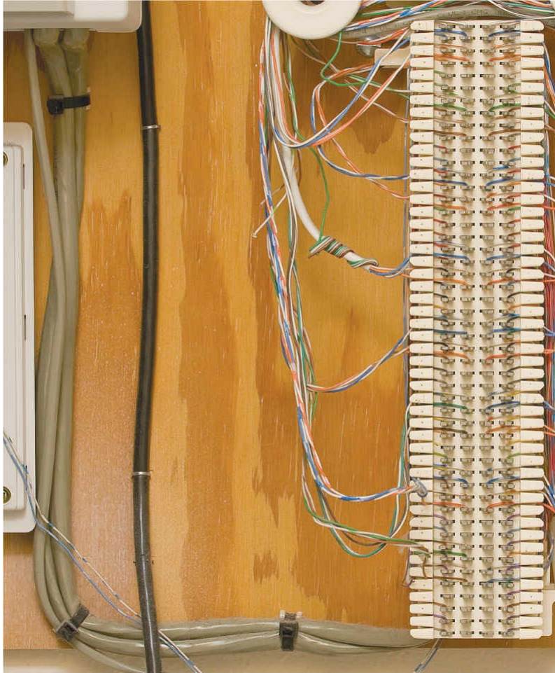
Figure 5-21 25-pair UTP cables running to local 66 block
