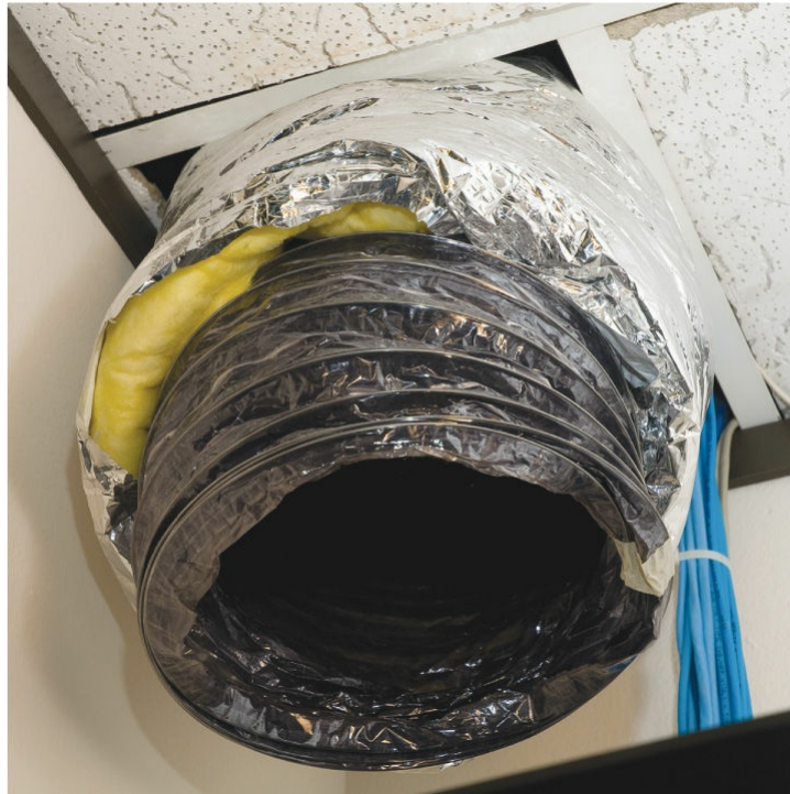
Figure 5-28 An A/C duct cooling a telecommunications room
