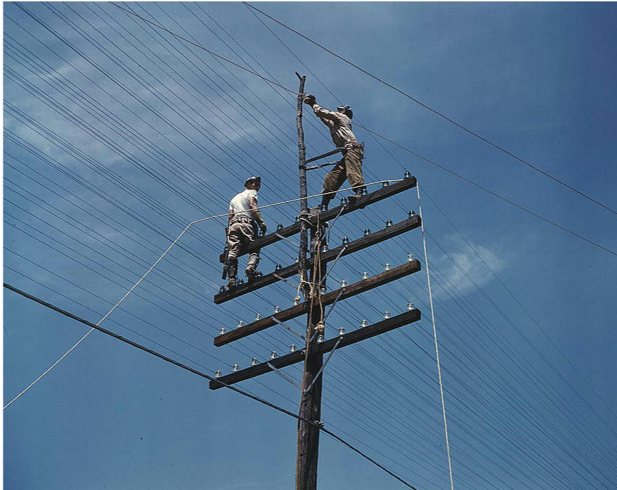
Figure 13-3 Now that's a lot of telephone lines!
