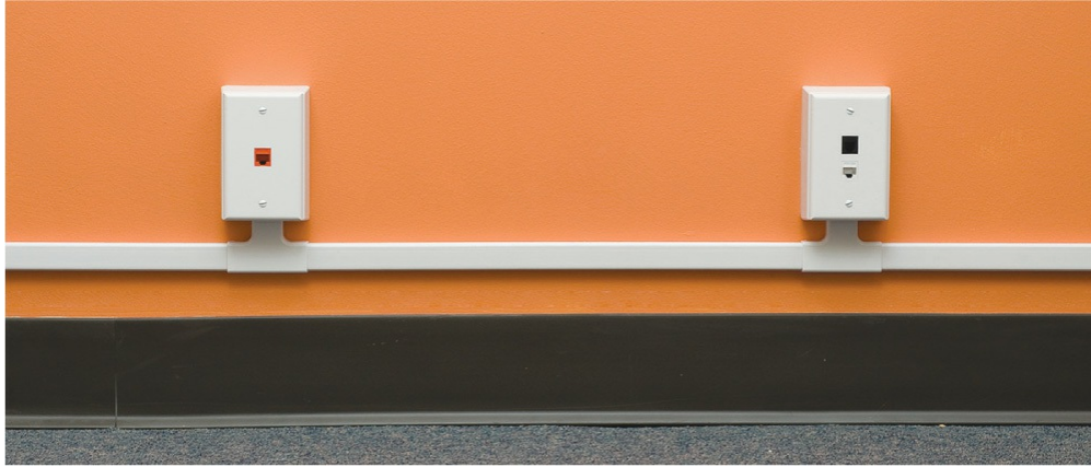
Figure 5-27 A typical raceway
